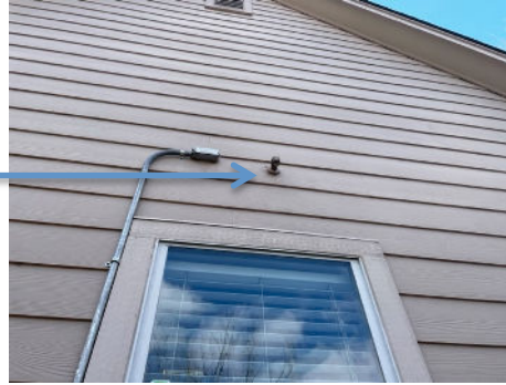
Secondary (emergency) condensate drain line
