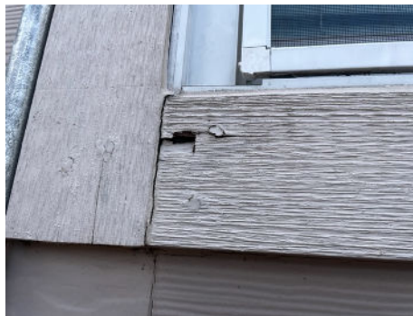
Minor decay on wood trim boards
