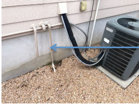
Primary condensate drain line
