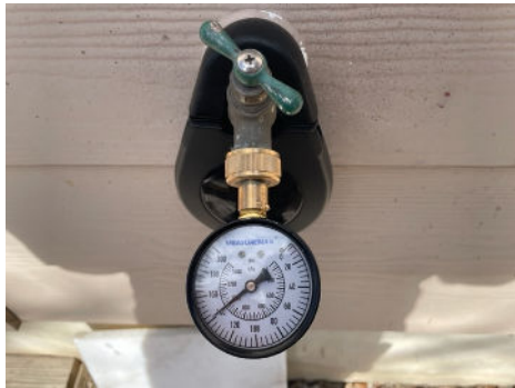
140 PSI- Recorded water pressure for the home
