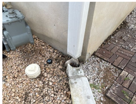
Missing elbow on gutter downspout
