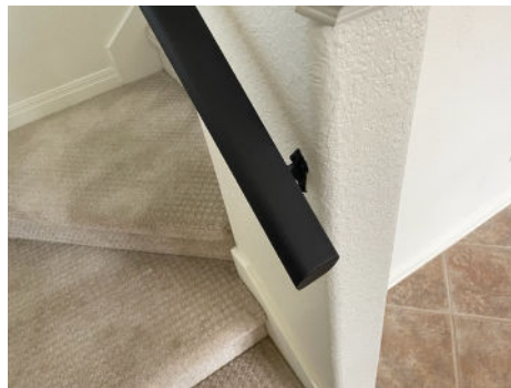
Hand railing not turned into wall at bottom
