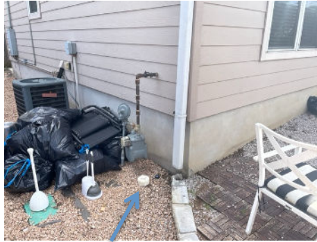
Main sewer cleanout for the home
