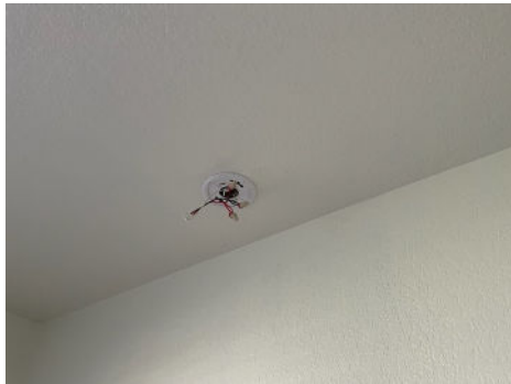
Missing smoke alarm in bedroom
