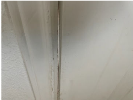
Weather-stripping not properly sealing
