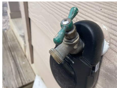
No anti-siphon device (back-flow preventer)
