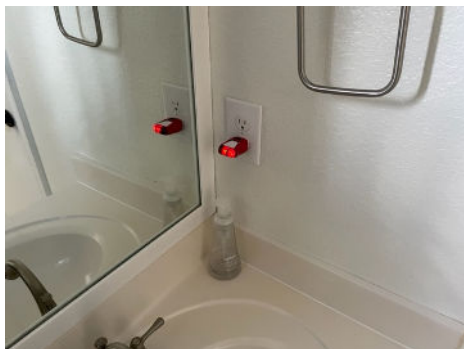
Loose wall outlet in bathroom
