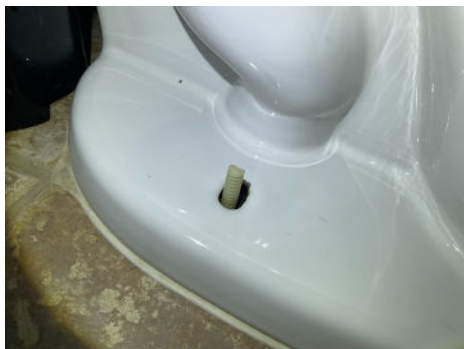
Missing anchor bolt on upstairs toilet
