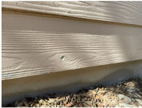
Nail popping in rear Hardie plank siding
