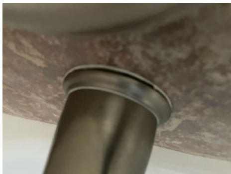
Voids in caulk seal on upstairs tub faucet
