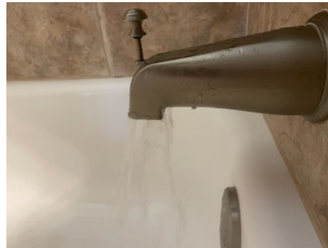
Faulty diverters in tub/showers
