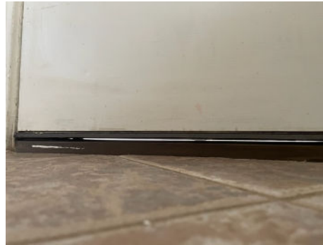
Front exterior door sweep not sealing
