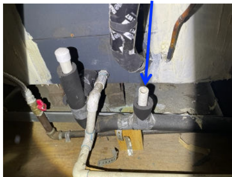
Hot water/bleach service to the primary condensate drain line
