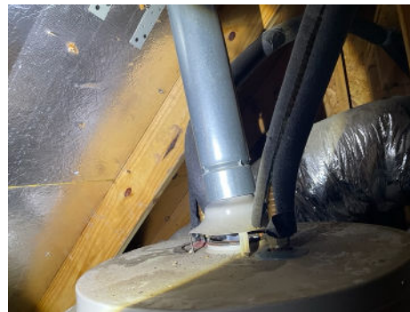
No 2-gallon thermal expansion tank
