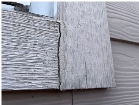
Minor decay on wood trim boards
